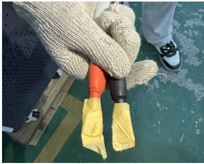
The insulation tape is wrapped around both ends of the positive and negative wires to complete the state
